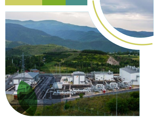
Metering Station (MS-1) Ardahan
